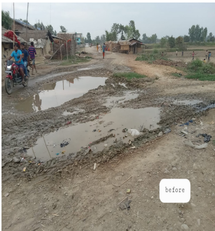
Before: stagnant water, no drainage on road.
